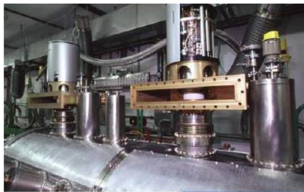
LEP coax to wave guide transition
